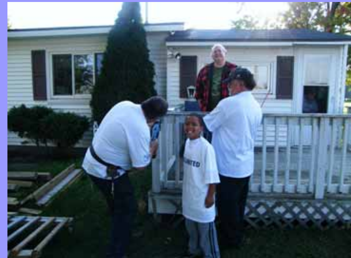
United Way of Bay County Labor volunteers building a new ramp for a local resident.
