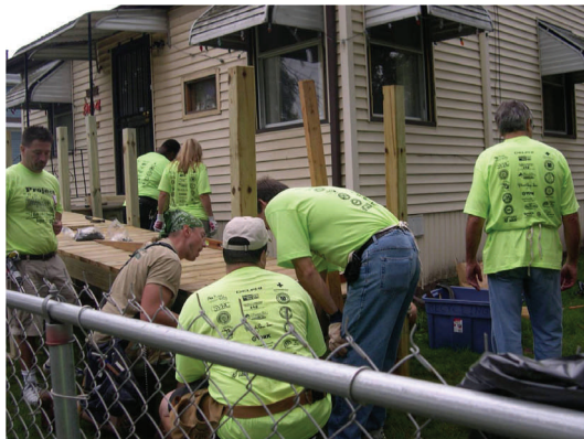
A mobility ramp being built by members of Carpenters Local 706, UAW Local 699 and Manufacturing Engineers from Delphi Steering, Saginaw, Michigan.
